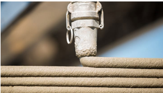
ICON's 3D-printer, Vulcan, draws the outline of the building one layer at a time. It can print up to 500 square feet in 24 hours. Credit: ICON
